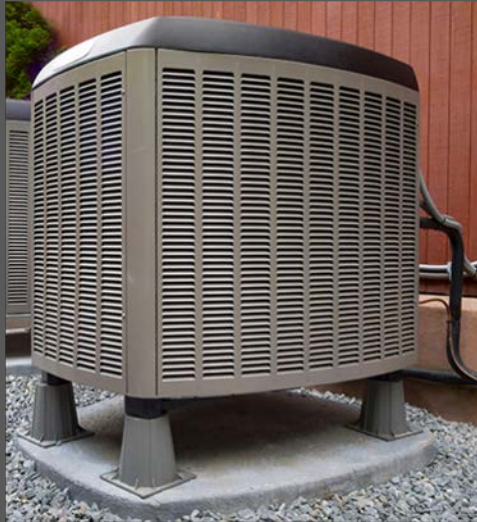
Heat Pump Space Heating/AC
